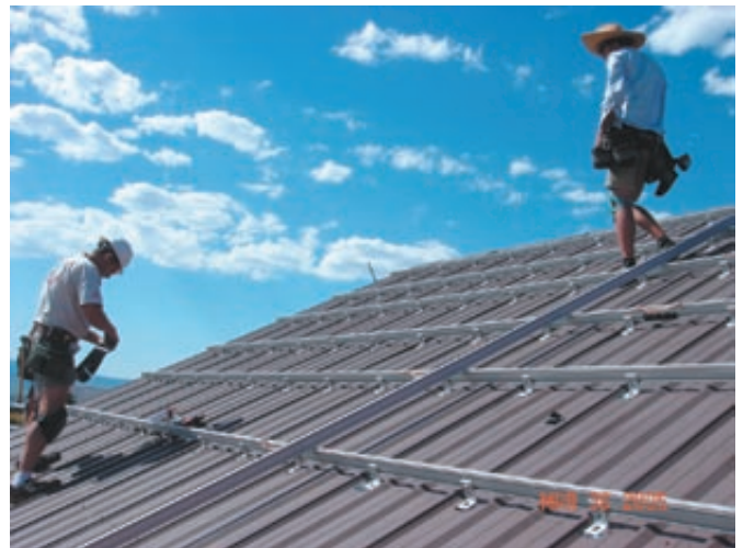
The solar array on the roof of the NOLS branch will offset 30-35% of annual electricity use.
