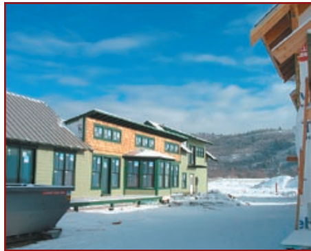
Mountainside Village in Victor, Idaho, is one of the GY-Framework registered pilot projects and a LEED-Homes pilot.
